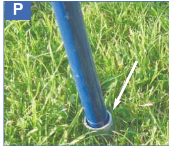
16. Make a pilot hole at the same angle as the back and sink in a ground leeve and drop rear leg into the leeve.
